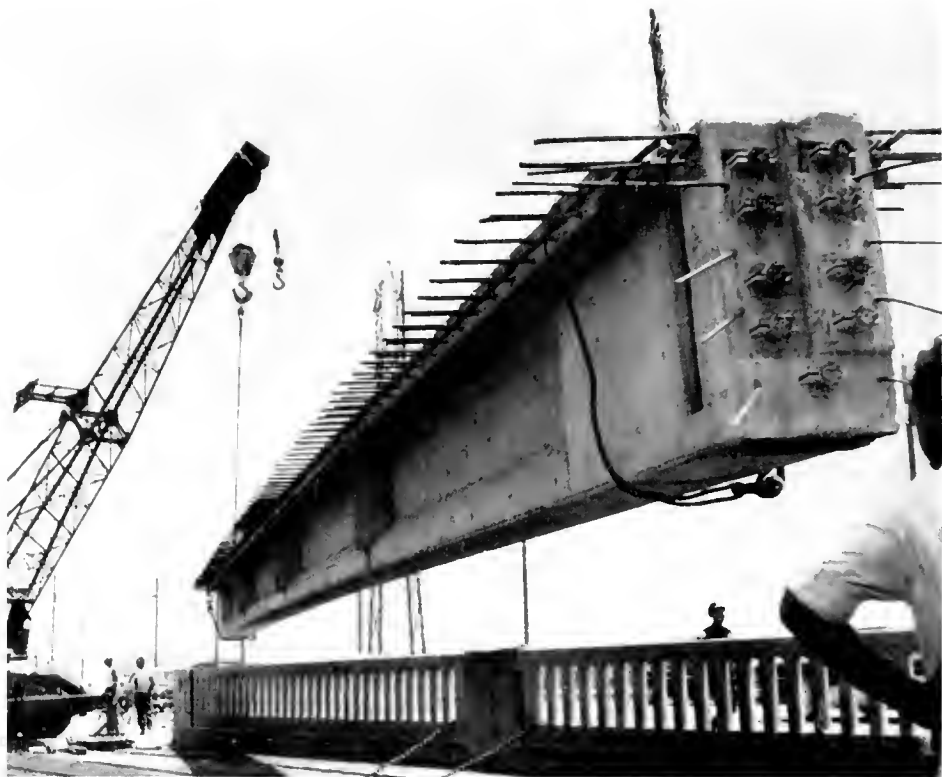
Photograph by Assistant Resident Engineer Tom Chew, showing prestressed precast reinforced concrete girder 80 feet long, weighing 24 tons, being swung into place to widen Santa Ana Freeway bridge over Los Angeles River.
